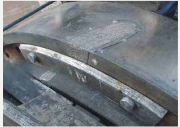
Kiln Tyre Crack Repair
